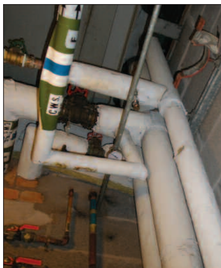
Well-lagged cold water distribution pipes.
