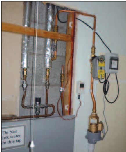
A flushing valve and timer set.
